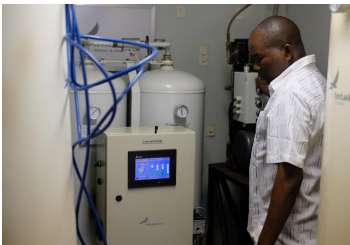
Oxygen medical gas is available to health facilities in multiple formats, including cylinders, concentrators, and central pipeline systems. Photo: PATH/Zachary Clemence.
